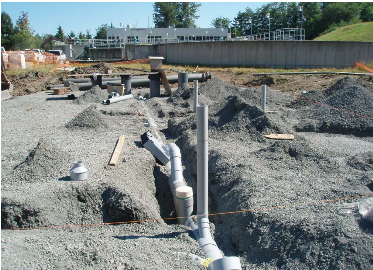
Saanich Peninsula heat recovery – Capital Regional District
