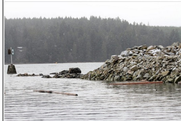
Approximately 150 feet of the breakwater at the Beachcomber Marina in Nanoose Bay has crumbled after gale-force northwesterly winds combined with a high tide battered the rocks on Sunday, Jan. 12. (Emily Vance photo)
