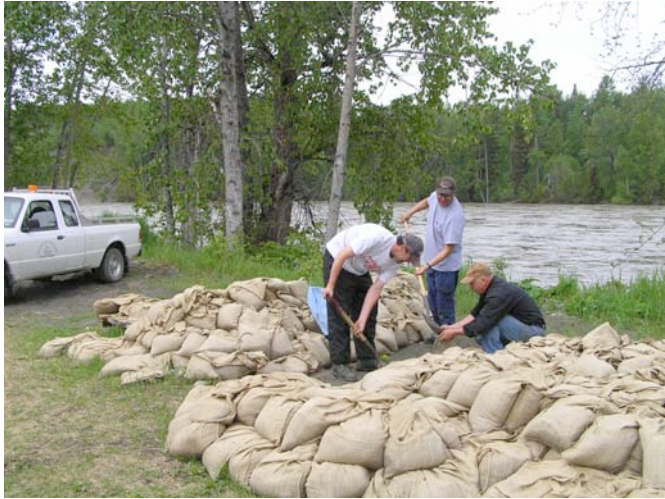
Staff from the Village of Hazelton engaged in sandbagging operations during the 2007 flood watch.
